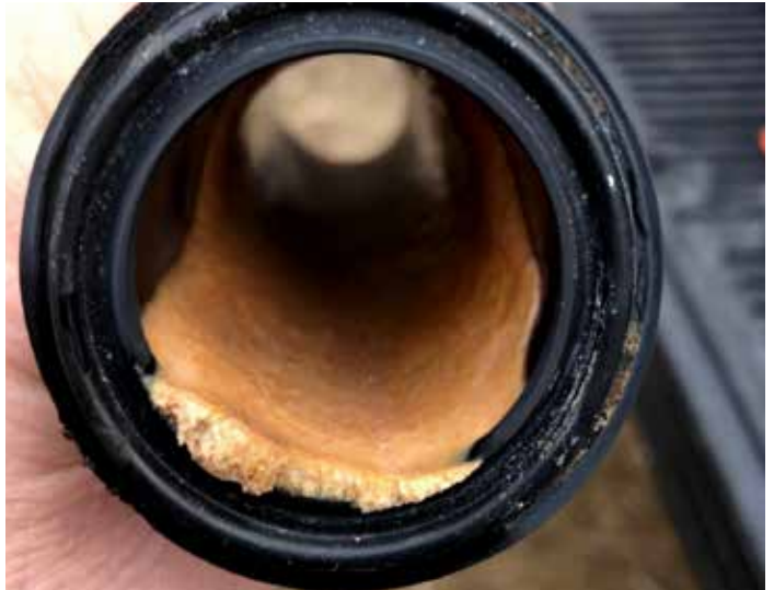
Severe example of biofilm build up in stainless steel pipe.
